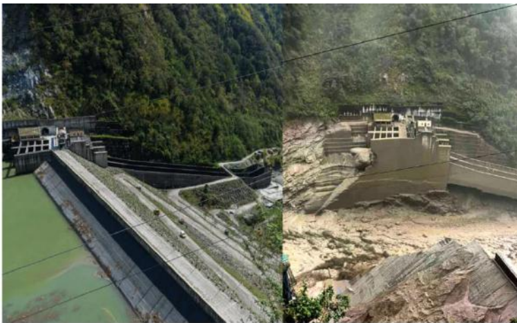
Before and after images of Chungthang Hydro-Dam in Sikkim
